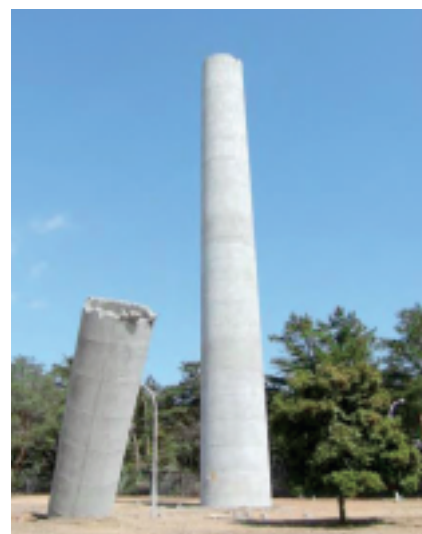
The chimney at JRR-2 was snapped in two by the earthquake on March 11, 2011.
